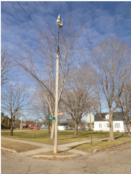
Existing Street Lighting
