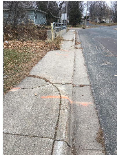
Cracked/ un-even Sidewalks
