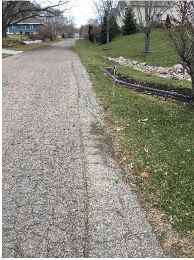
No Curb & Gutter
