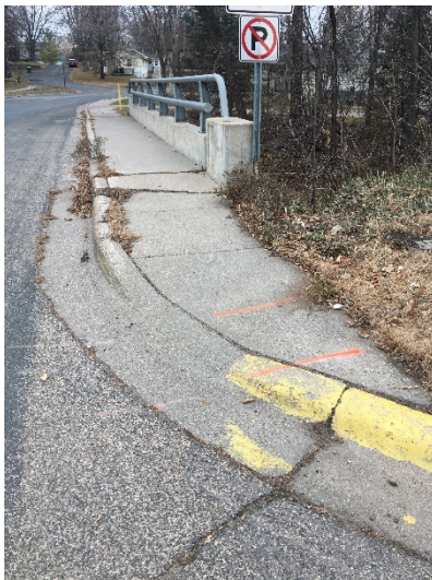
Non-compliant Pedestrian Ramps
