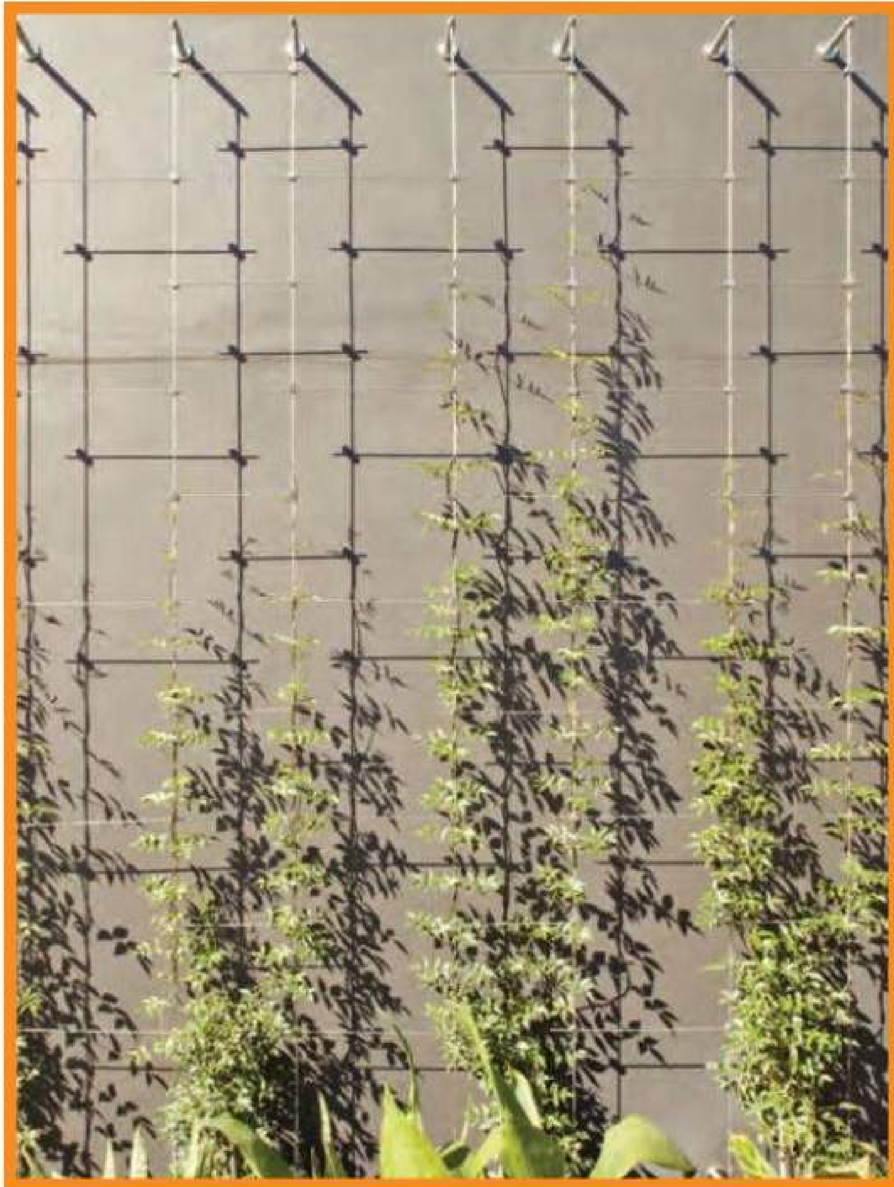
Green wall, cables with vines.
