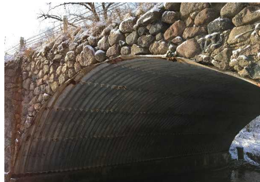
Failing stone headwall at steel arch bridge
