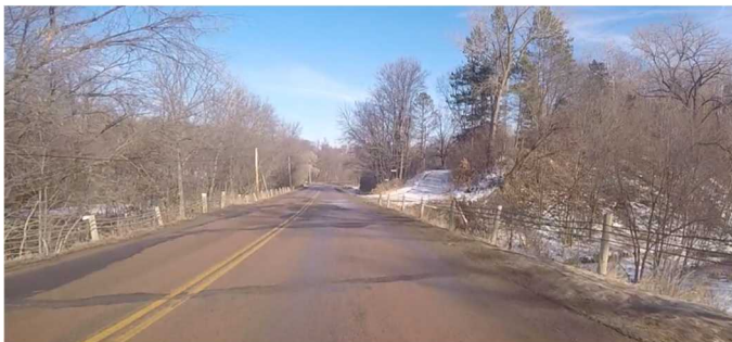
Failing Bridge Guard Rail
