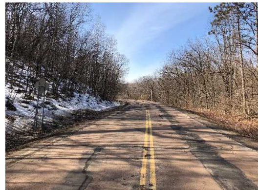
Extensive Roadway Cracking
