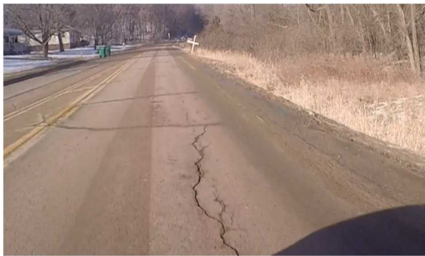
Longitudinal and transverse cracking
