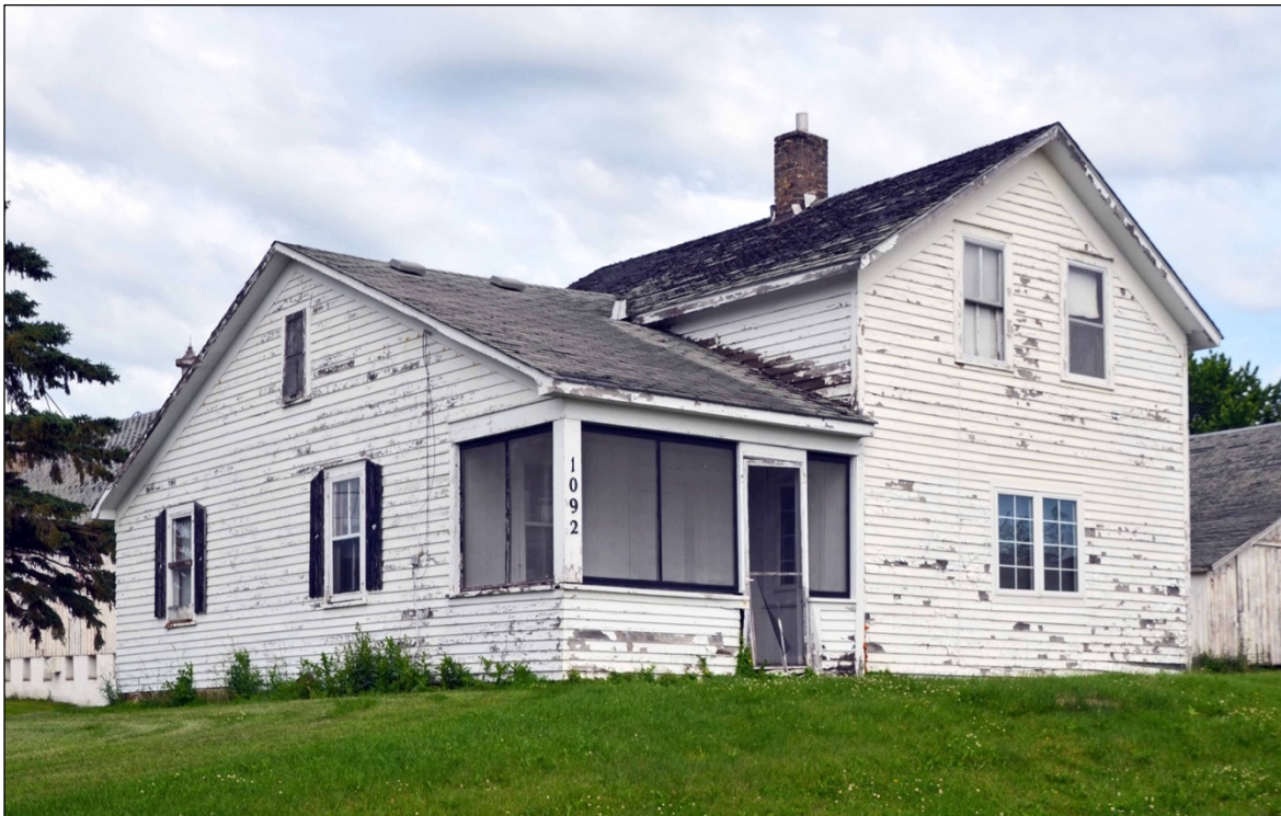
Photo 16. South and east elevations. Clapboards on the east wall of the original section are continuous, suggesting that the house was at least partially re-sided when the original door and window openings were filled in.
