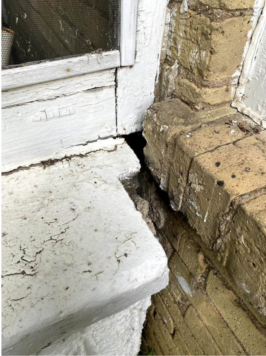
Porch pulling away from house due to deteriorating foundations
