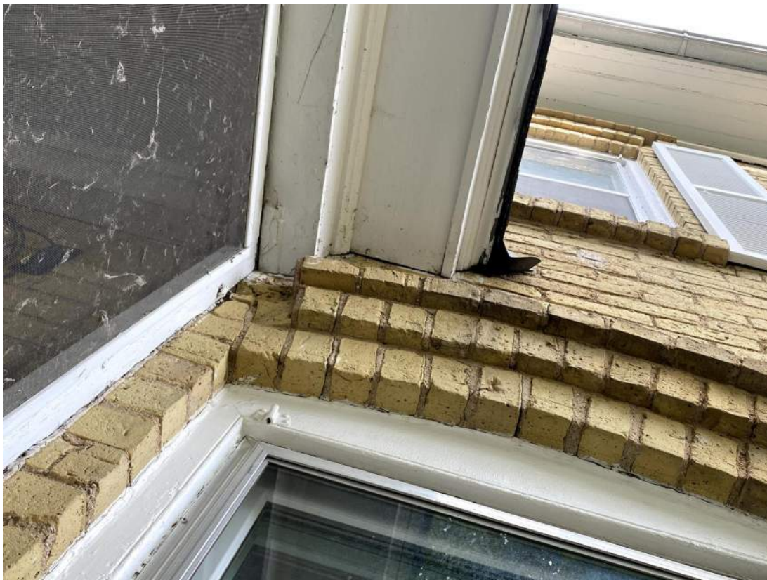
Damage to corbelled brick detail due to porch construction
