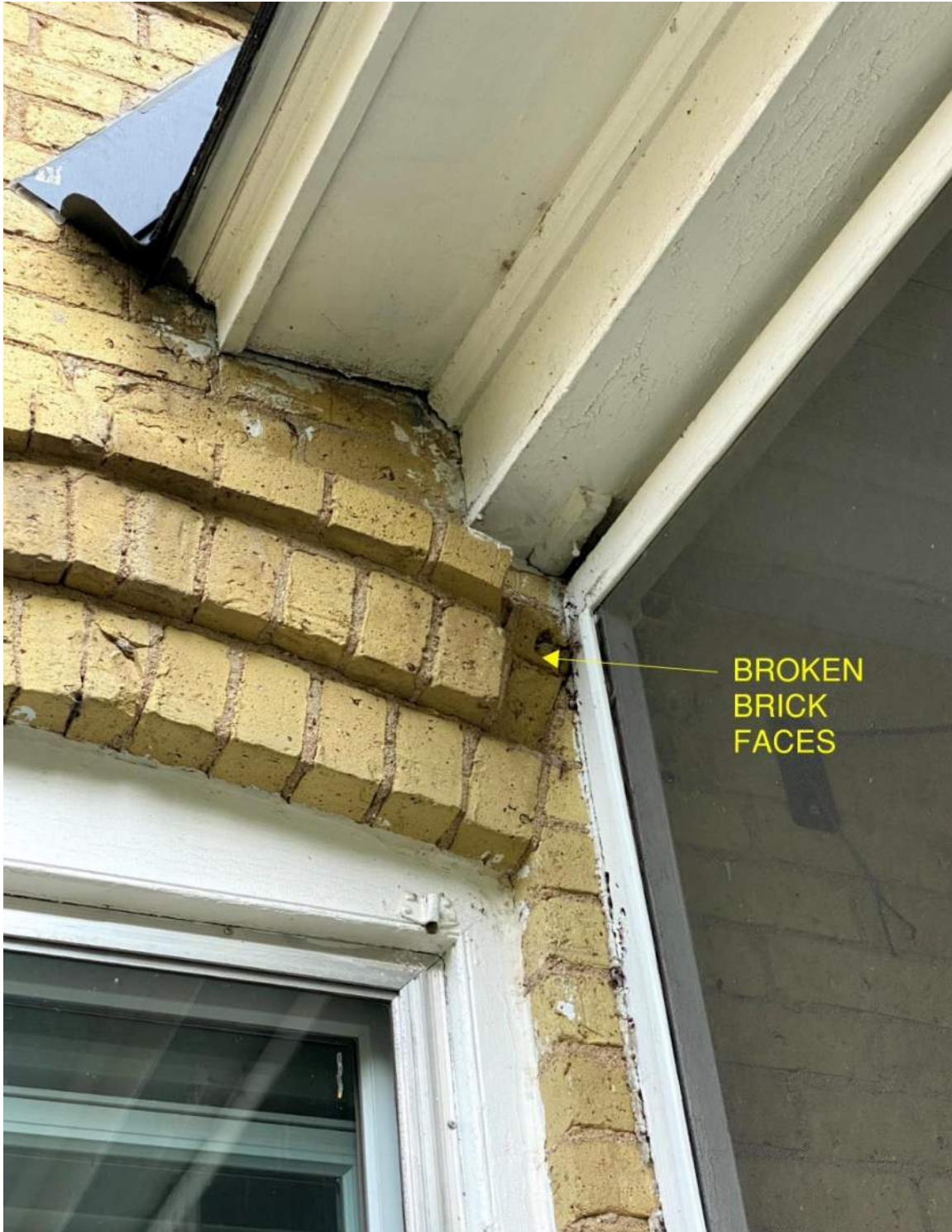
Brick ornament was crudely destroyed to install porch details.
