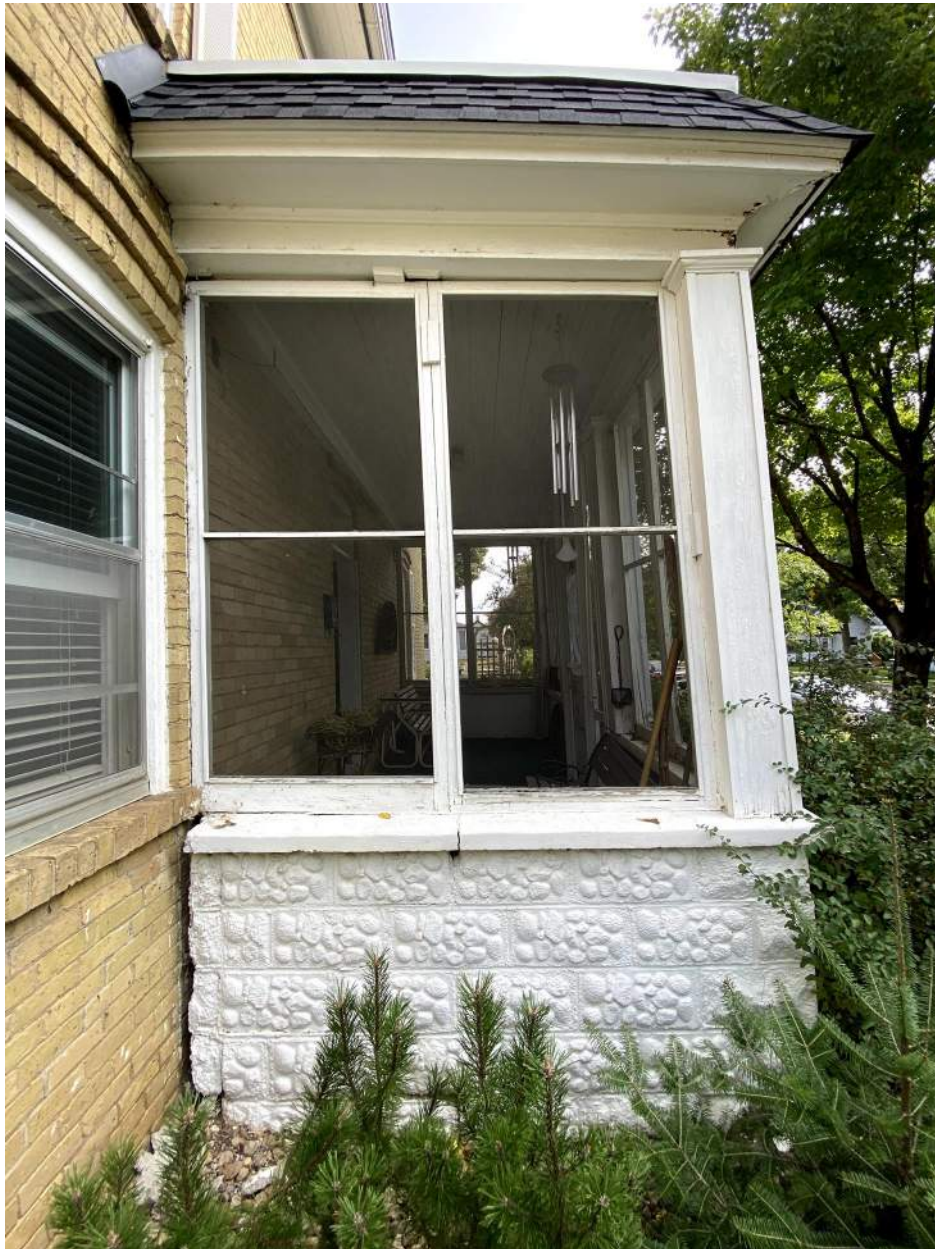
Note lean in porch columns as south foundation pulls away from house
