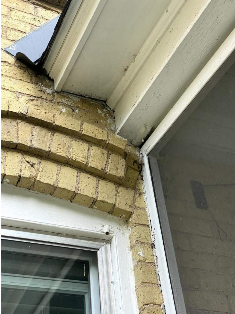
Damage to corbelled brick detail due to porch construction
