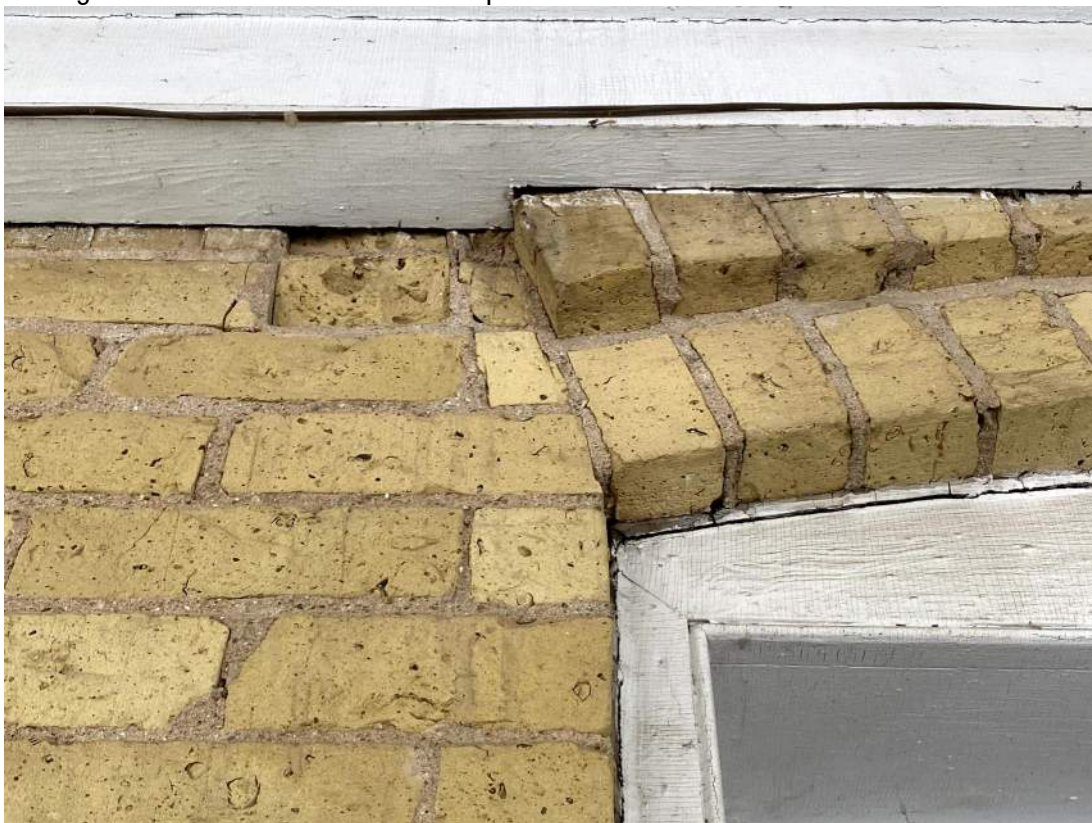
Damage to brick above entry door
