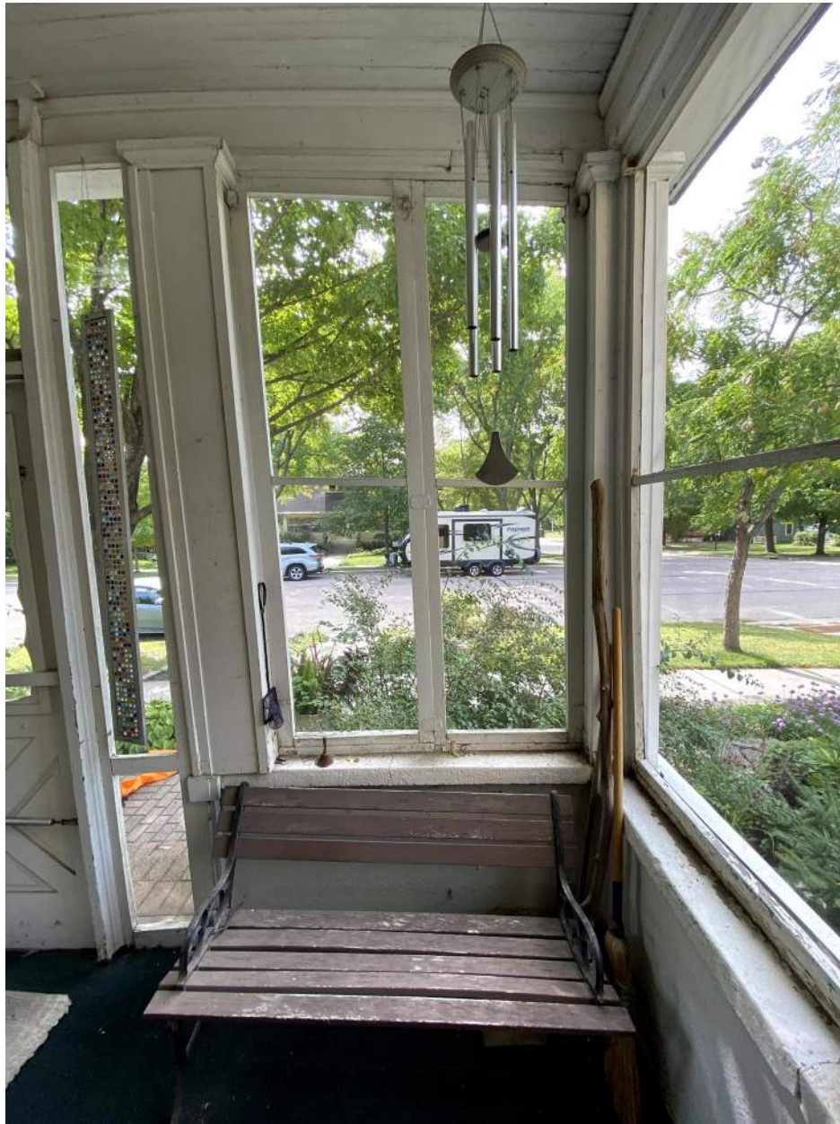
Note sagging floor structure
