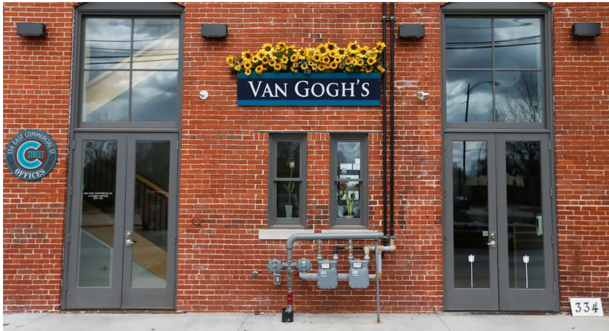
Wall-mounted fixtures are installed alongside doorways in the above example of a rear business entry.
