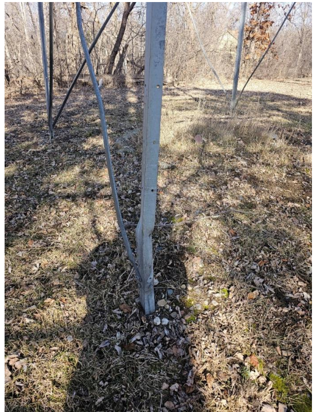
View of base looking NE noting buckled leg member.
