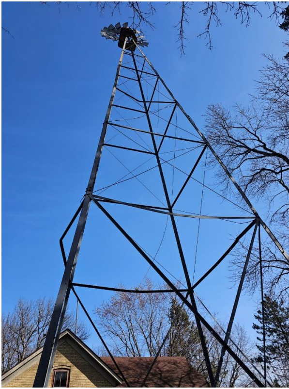
View looking east noting buckled cross members.
