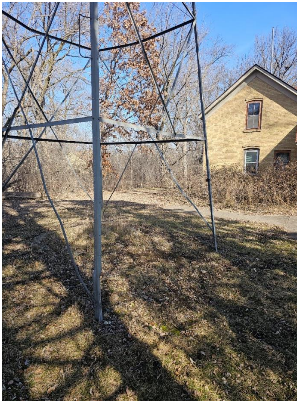
View looking NE noting missing & buckled members, as well as proximity to house.
