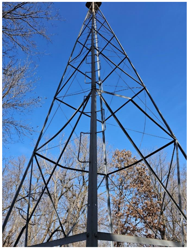
View looking NE noting buckled cross members.
