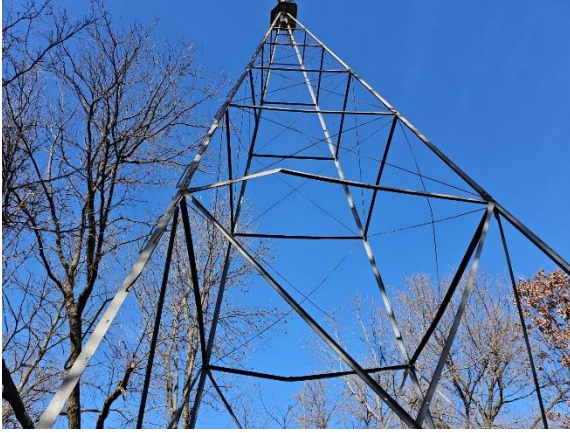
View of upper portion looking SW noting buckled members.
