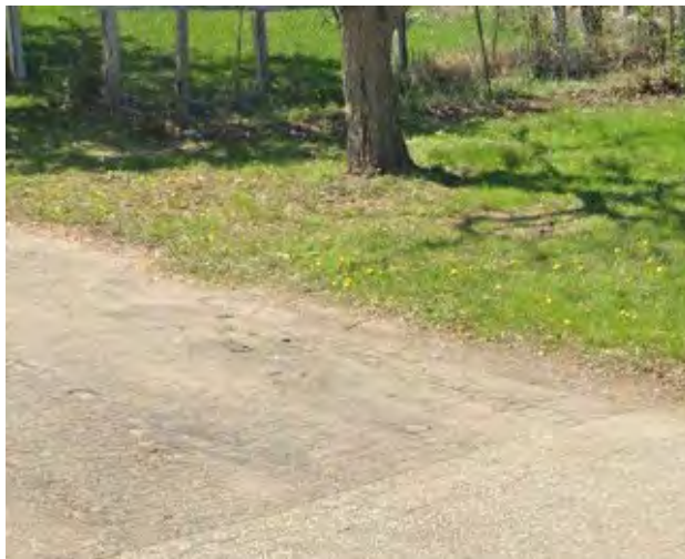
No Curb and Gutter
