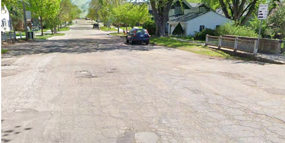
Distressed pavement and poor drainage
