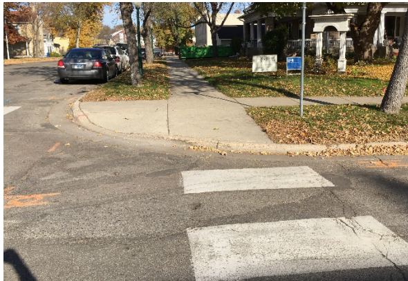
Non-compliant Pedestrian Ramps
