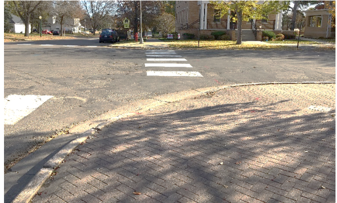
Non-compliant Pedestrian Ramps
